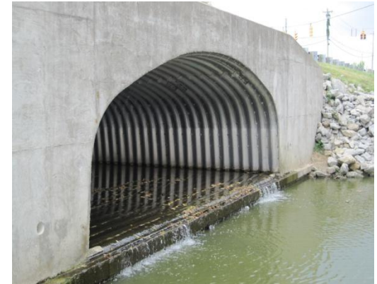
Above: Figure 2. One of the many aluminum box culverts I collected data from
