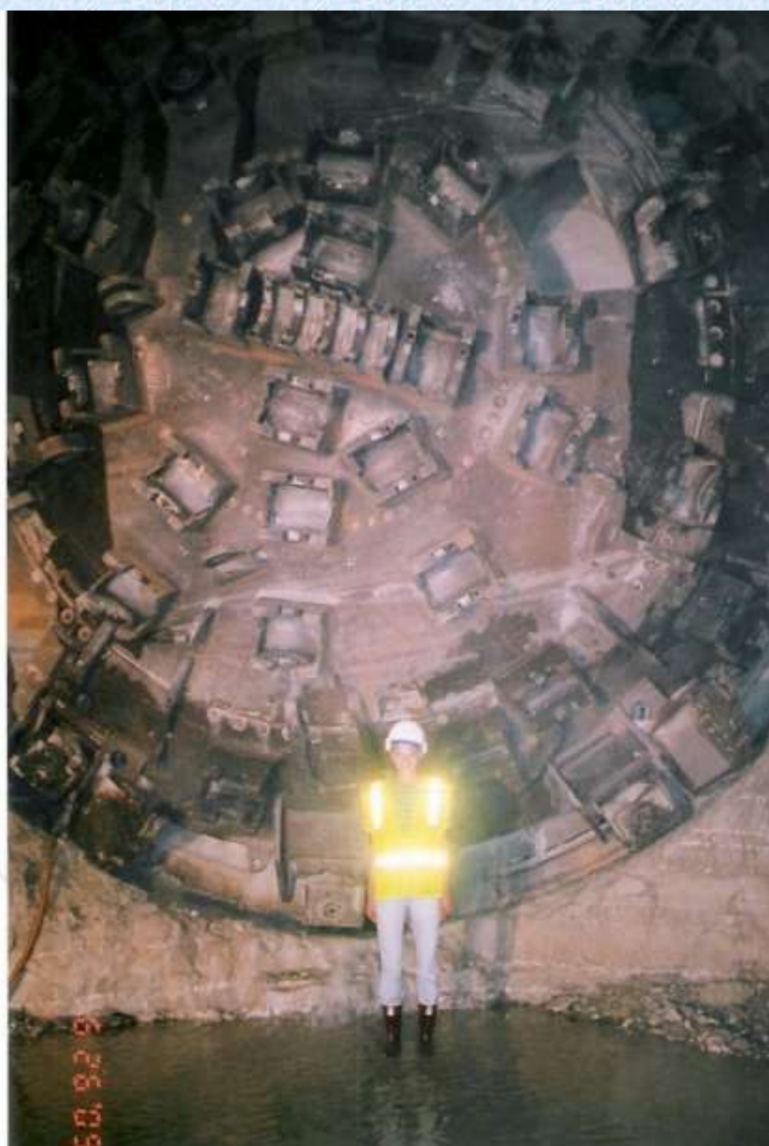
Figure 1. A picture of me inside a sewer during its construction. The sewer is 17 feet in diameter and is 350 feet underground. There is a boring machine behind me..
