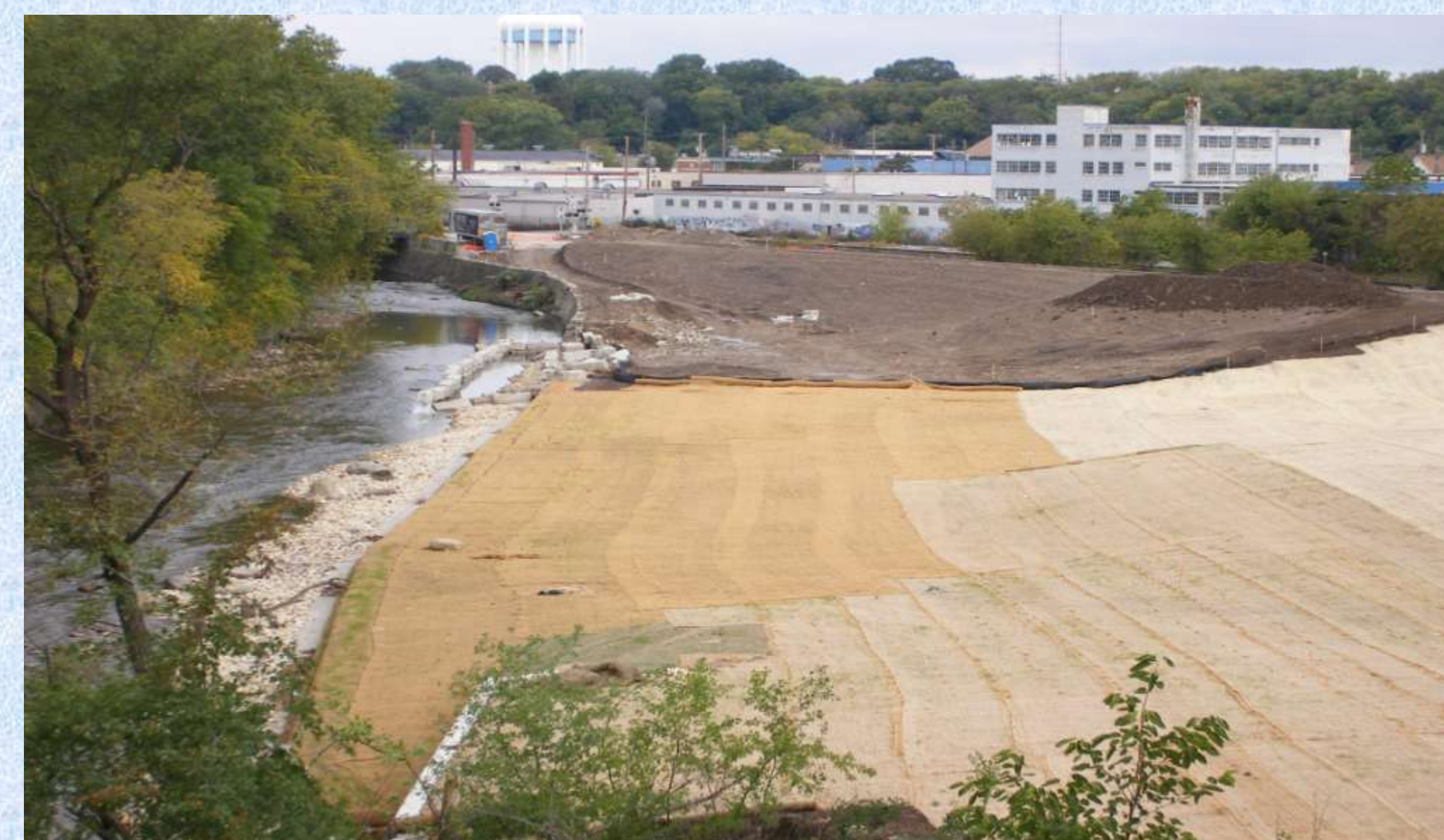
Figure 3. The soil contamination project after the contaminated soil was removed. This picture shows the current restoration of the river bank. In the spring, grass will grow up and hide the fabric.
